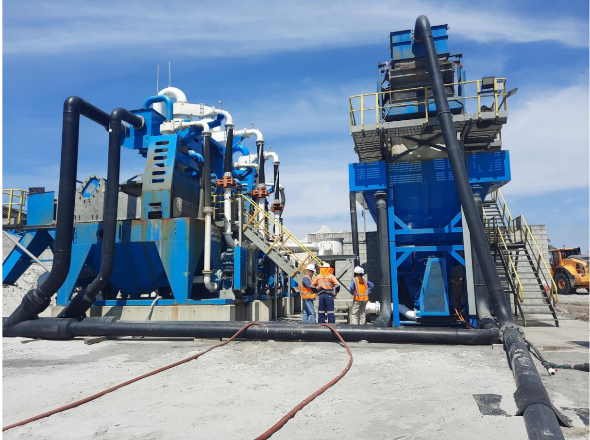
Plate 2 – Primary wash-screen process on right and dewatering units on left
