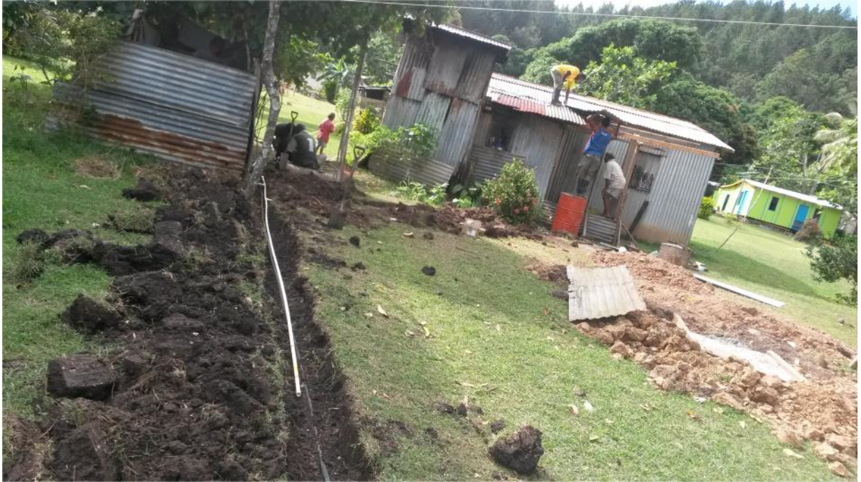
Figure 5: Water line being installed to the Ono Island building shown in Figure 4.
