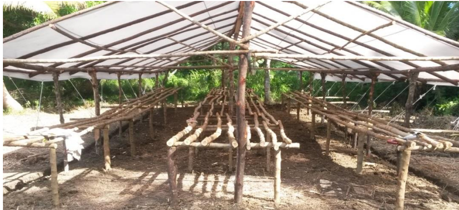
Plate 2 – Core handling building being constructed in preparation for Ono Island diamond drilling program
