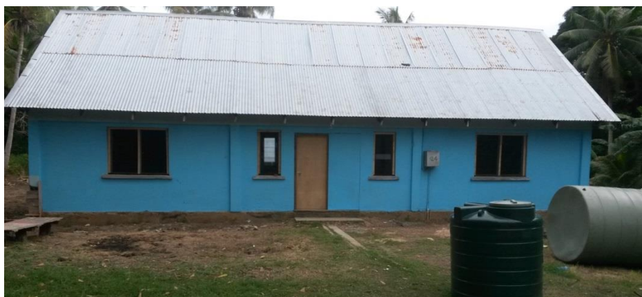
Plate 1 – Refurbished building that will provide office and accommodation for the geological team on Ono Island
